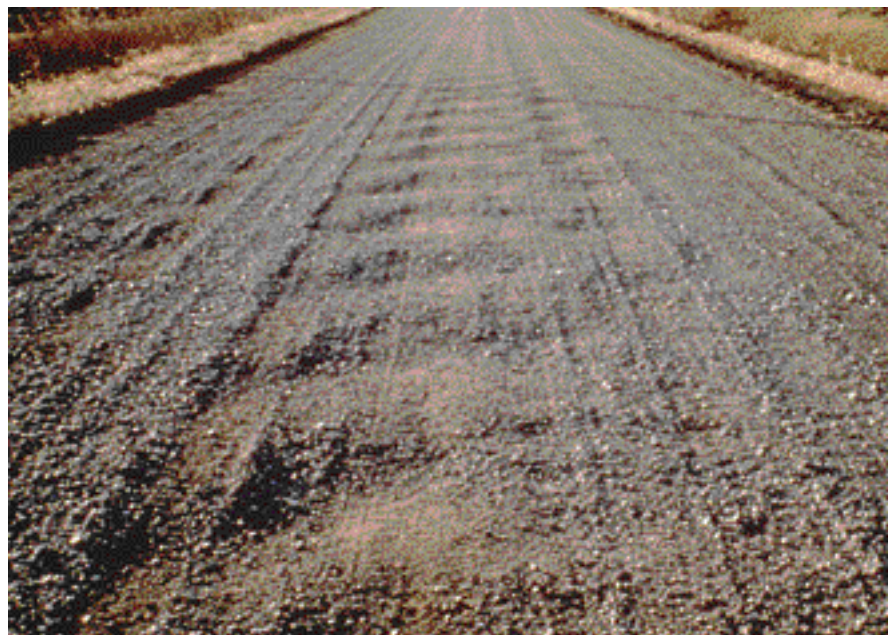
This type of washboarding appears at an angle across the roadway with ridges and depressions two to three feet apart. It is caused by excess grader speed.
