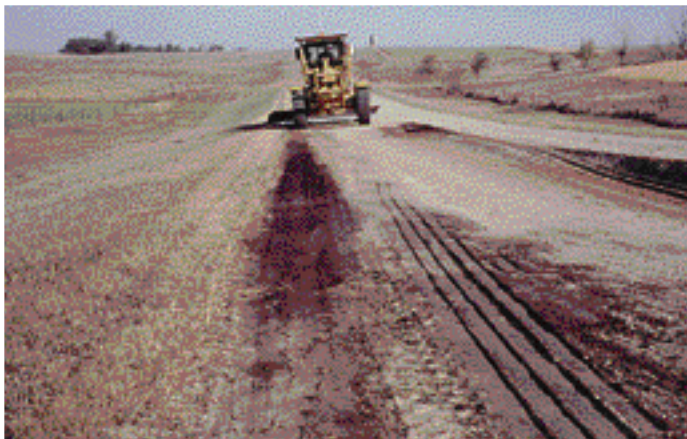
The existing secondary ditch is then cut slightly deeper and the material is placed in the roadway.
