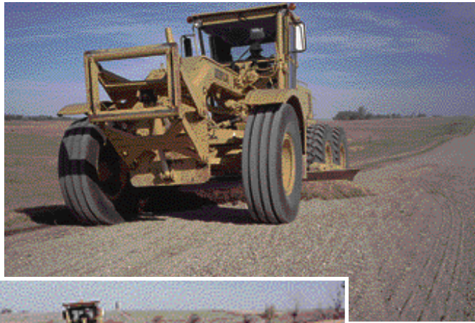
The existing surface gravel is cut loose and windrowed to the opposite side of the road.
