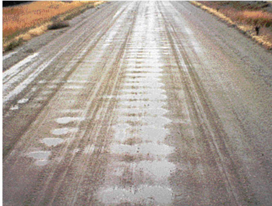
A road that lacks good crown. There is also centerline corrugation (washboarding), a problem that will grow worse when there is inadequate crown.
