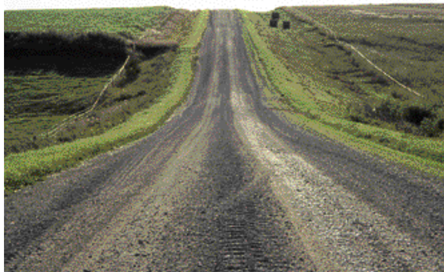
A gravel road with a 26-foot driving surface, yet everyone drives in the middle. The primary reason is excessive crown.
