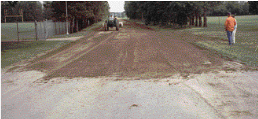
Another washboard-prone area is at the transition from paved to gravel sections as shown in this photo.
