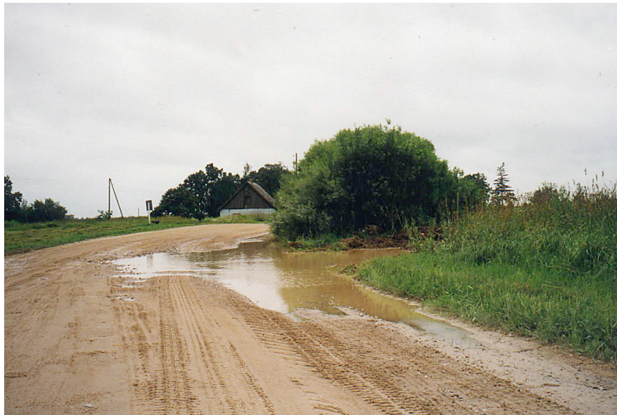
Lack of a roadside ditch has caused major drainage problems on this road. (Courtesy of Road Research Ministry of Roads/Transportation, Sweden)
