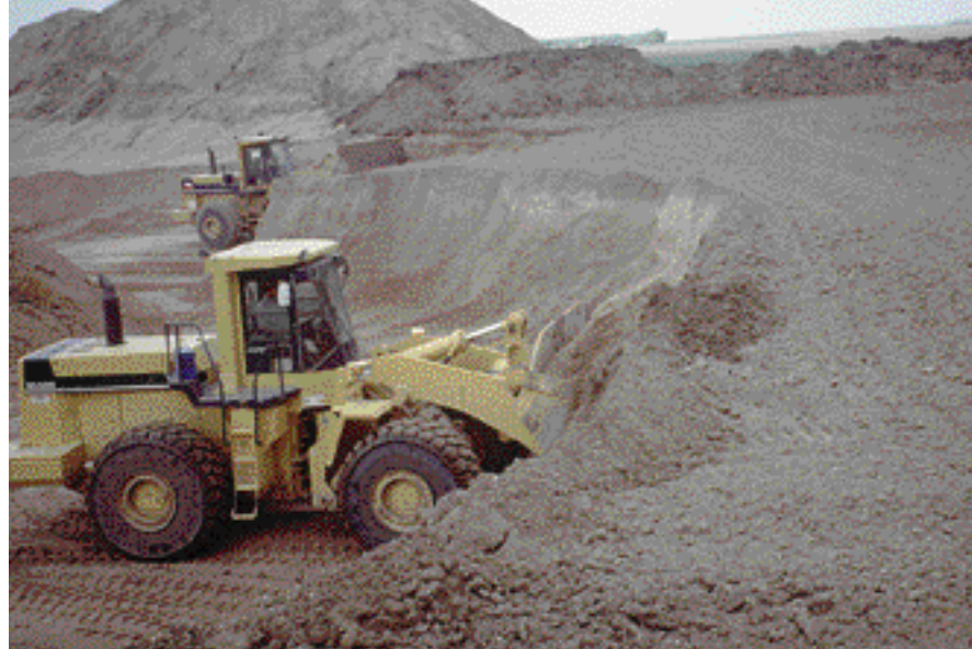
A very good example of working a gravel bank. Large loaders are being used to feed a crushing plant. Notice the good effort to work a broad area of the gravel bank. The operator virtually never takes a bucket of material from the same spot twice. This assures a good blend of material going into the crusher.
