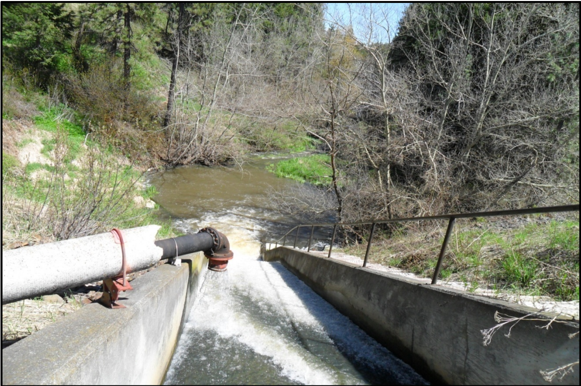
Photograph by EPA on May 18, 2011 looking at outfall 001 for the wastewater treatment plant. Effluent flows approximately ¼ mile east from the plant to the spillway from Lake Winchester to Lapwai Creek.
