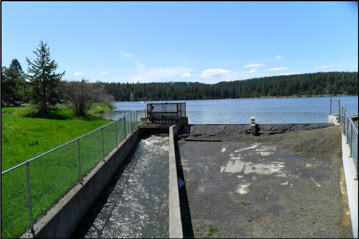
Photograph by EPA on May 18, 2011 looking at the spillway from Lake Winchester to Lapwai Creek.
