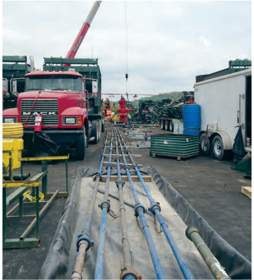
Completion equipment at a gas well.
