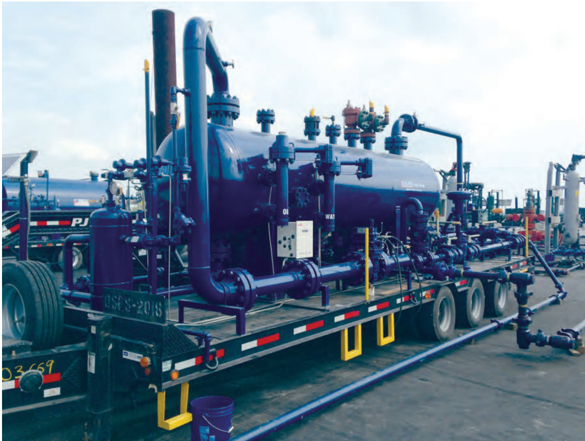
Equipment at a gas well.
