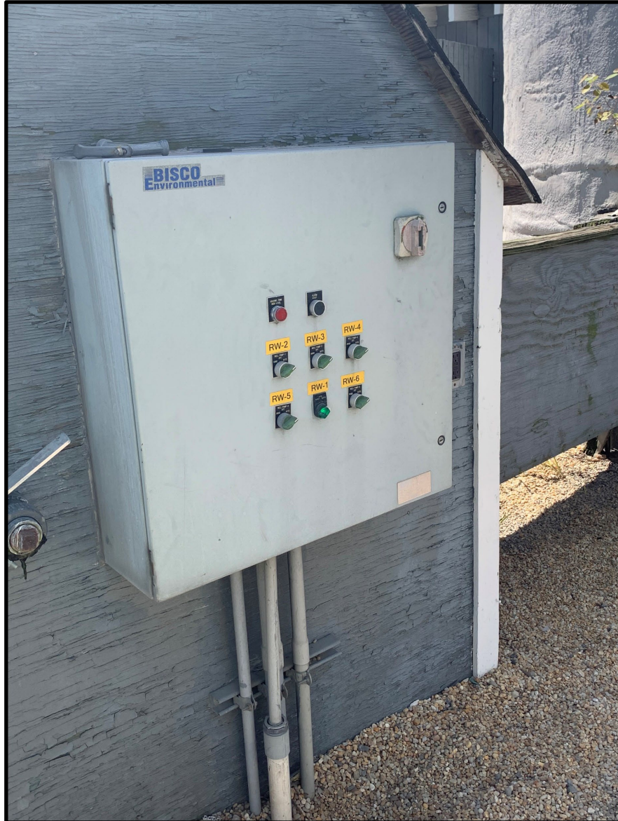
Picture 3: Storage Tank Control Panel
