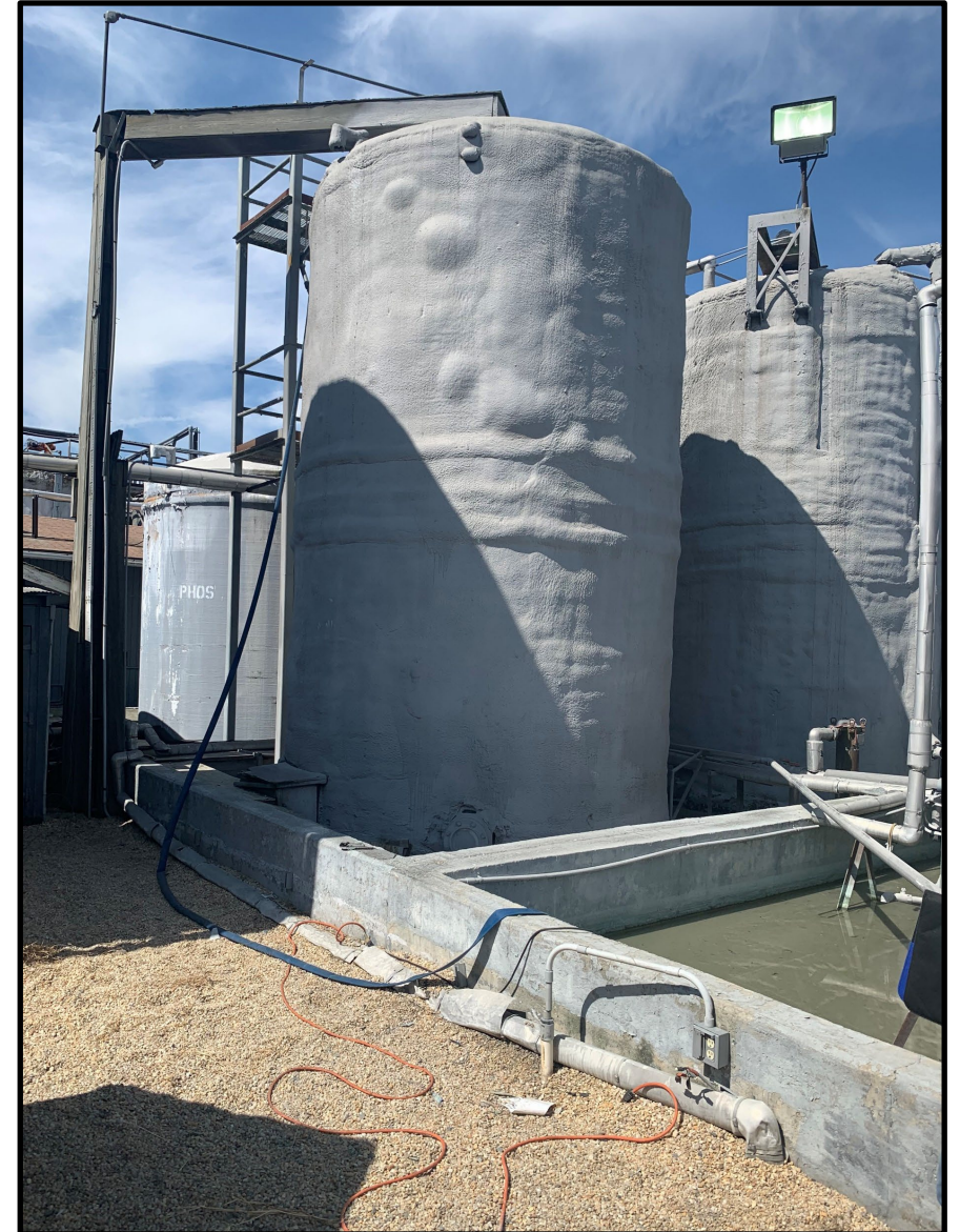
Picture 4: Storage Tank
