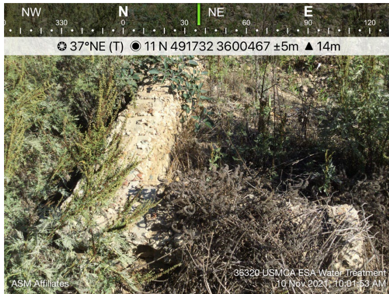
Figure 16. The retaining wall is located on Smuggler's Gulch's west bank near the northern end of SDI-11948H.
