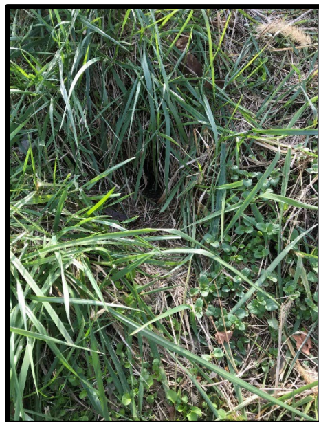
Picture 16: Holes in the Northern edge of Old Landfill Area, facing the south.
