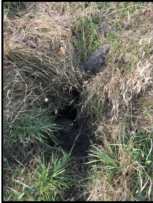
Picture 13: Holes in the Northern edge of Old Landfill Area, facing the south.
