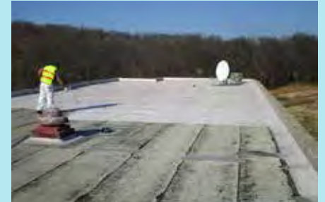
Crews install a cool roof at Browne Education Campus Photo Credit: Paul Lanning, Lightbox Energy
