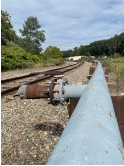
5. Possible Southern End Crude Unloading Area pipe valves
