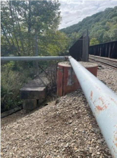
4. Possible Southern End Crude Unloading Area pipe bend
