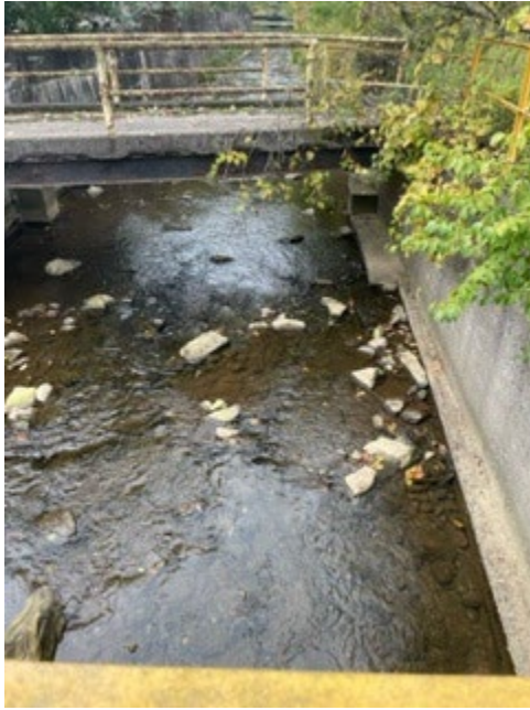
16. Cherry Run abutment cap remnants– looking down from railroad bridge facing downstream
