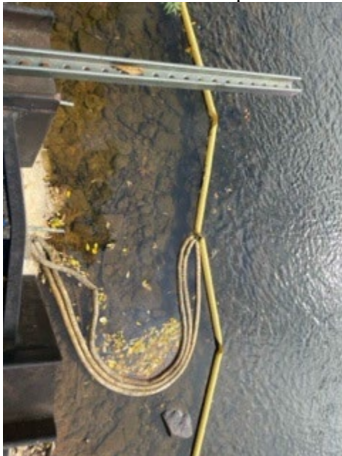
19. Outfall W area seep from above
