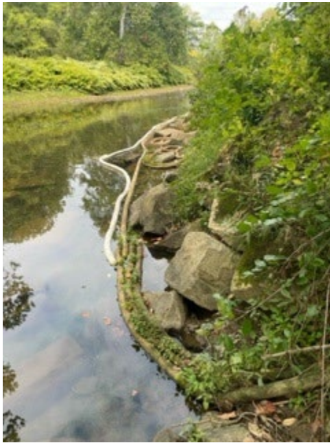
6. Southern End Crude Unloading Area seep - close
