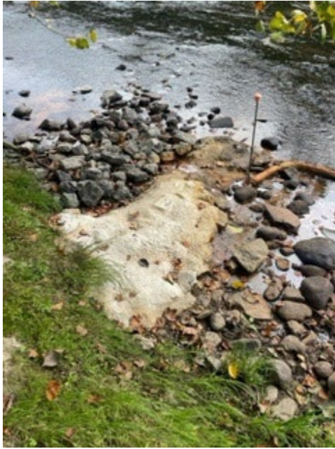
25. prior pipe sealing attempt to reduce seep
