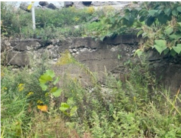
31. deteriorating retaining wall
