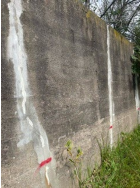
27. typical previous seep remedy approach – seal breakthrough area
