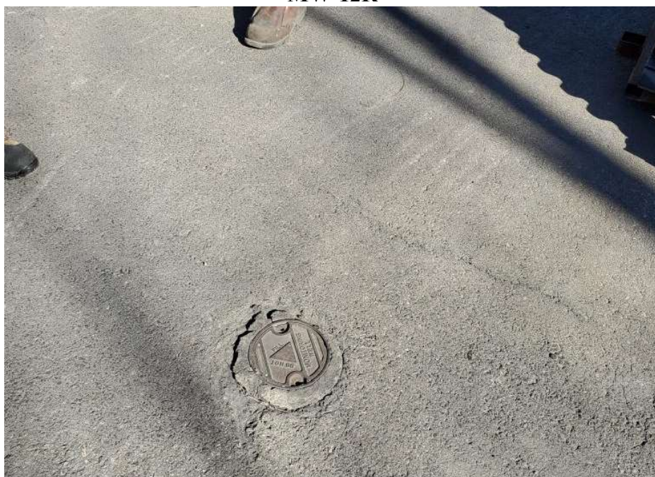
At MW-12R. Monitoring well not labeled with well number.
