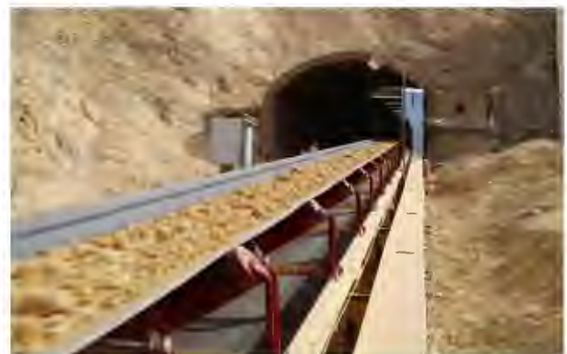
Image 4 – Photo showing a conveyor system. Temporary conveyor system fabrication may vary.
