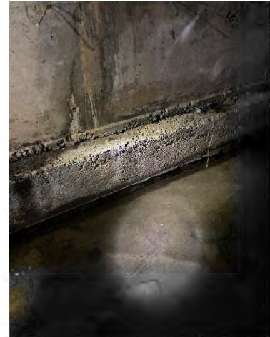
Image 3 – Scour at the Foundation
