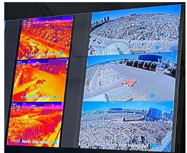
Figure 4: A control room monitor depicting video feeds from several remote thermal imaging (infrared) and regular cameras at the facility.
