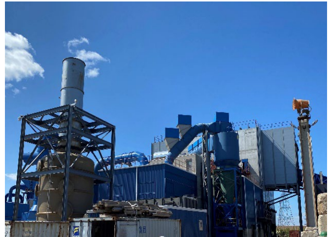
Figure 2: An enclosed metal shredding facility equipped with a thermal oxidizer and water cannon.
