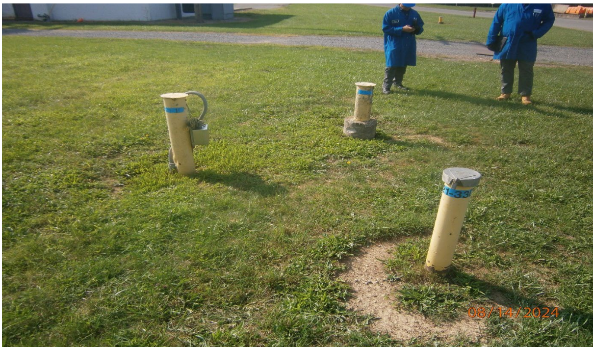
Nested Monitoring Wells
