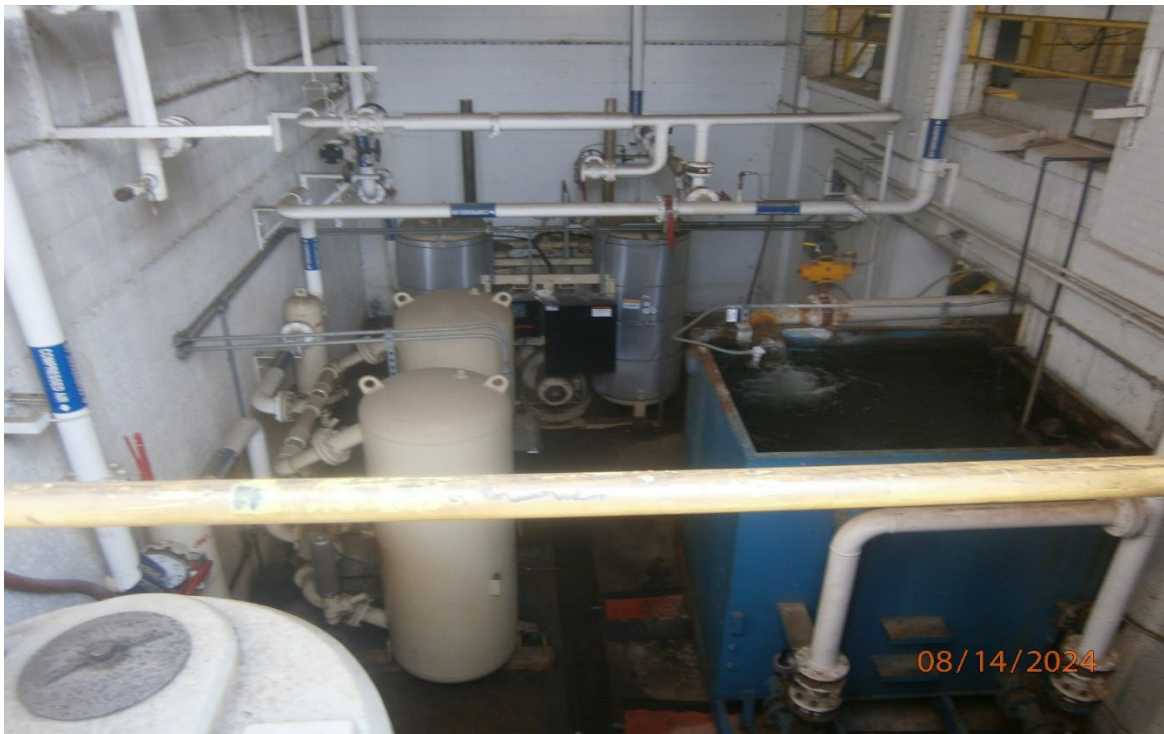
Active Carbon Groundwater Treatment System
