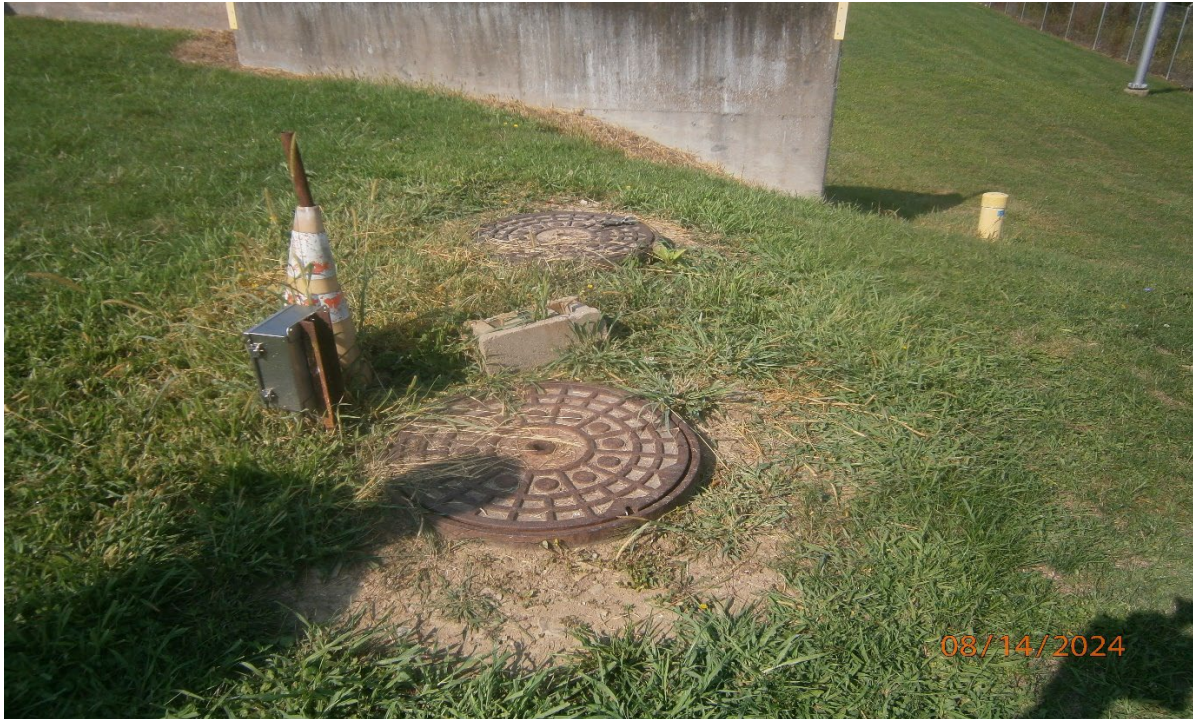
Manholes to route purged water to the onsite wastewater treatment system.
